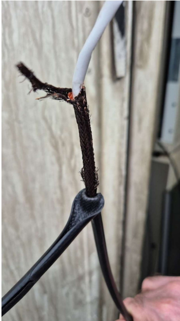
Figure 3 The coaxial cable damage
